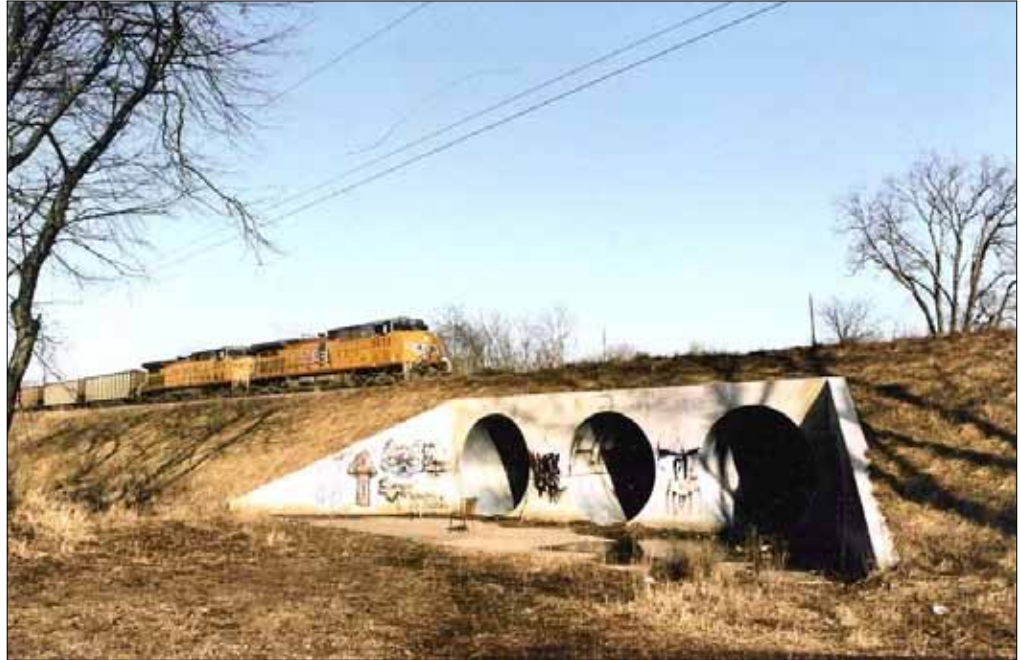
Top Photo: The Sac & Fox Trail may cross under the Union Pacific tracks, through one of these culverts.
